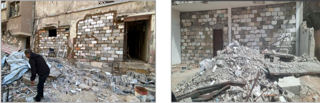
Figure1 Sealing off missing wall parts with reclaimed cement blocks to close the openings
